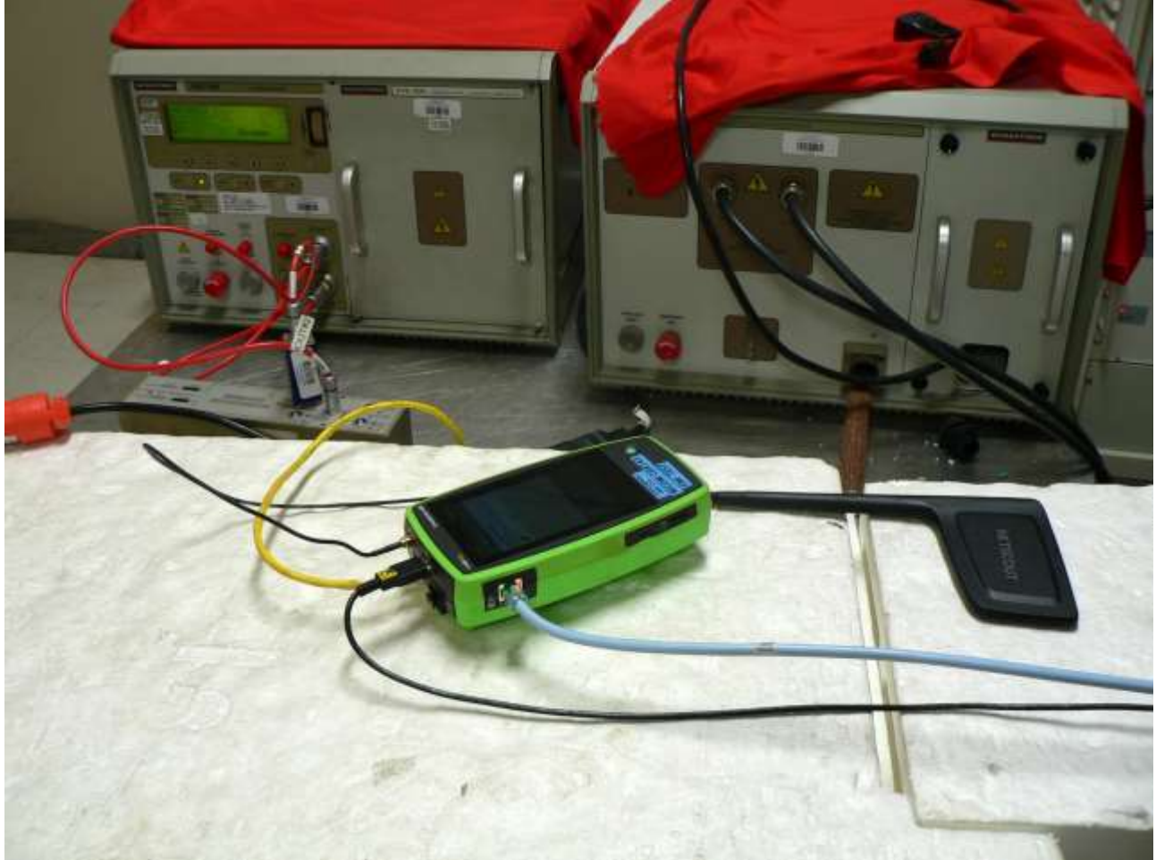
Battery Test Port:
